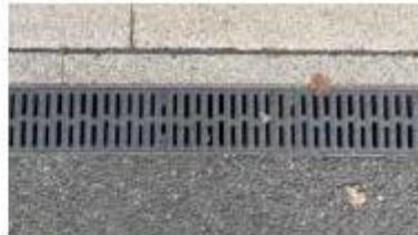
2 Existing metal grating
